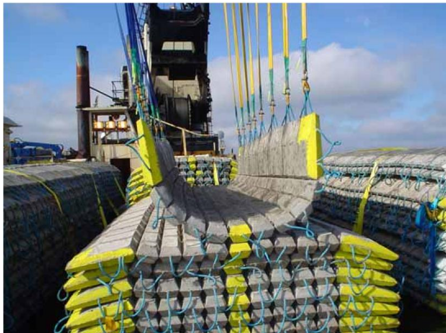
Figure 5 – Pick up of single concrete mattress prior to over-boarding. Note: Organised stacks allowing clear stretcher route access
