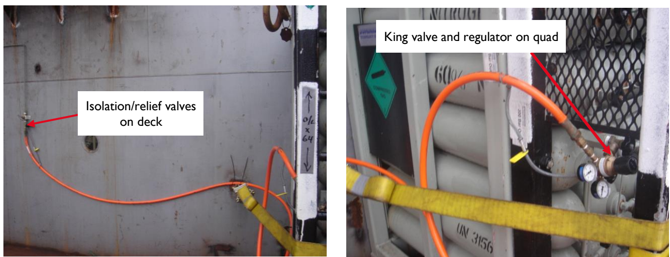
HP charging hose from supply quad used for decanting
